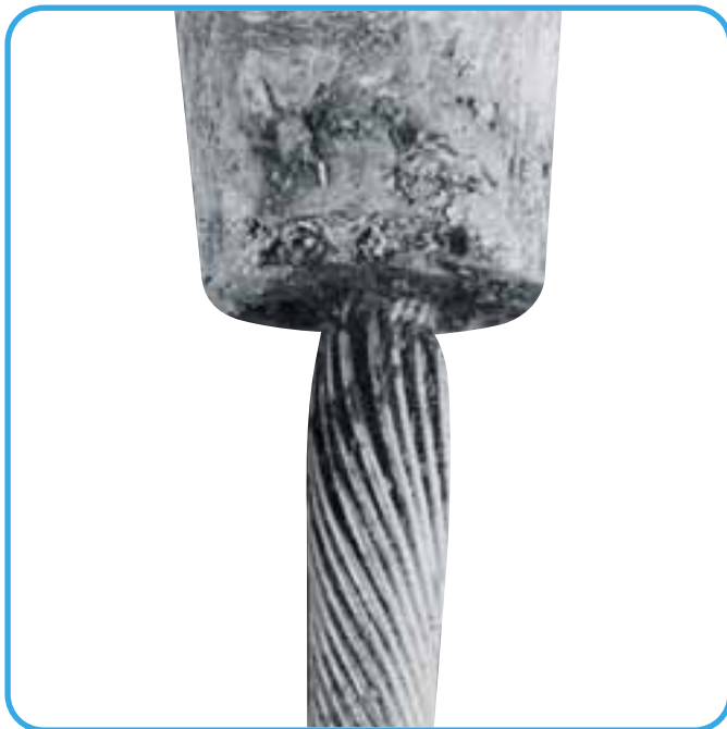
Figure 13: Typical example of the swelling of stainless steel rope due to Crevice Corrosion.
